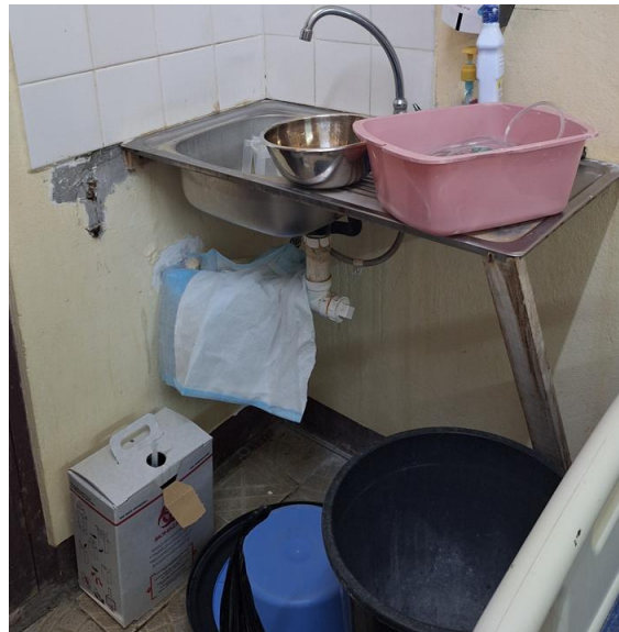
Figure 8-9: Showing Sink in Operating Room flowing into outside drains
