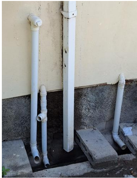
Figure 8-8: Showing Sullage flow into outer drains
