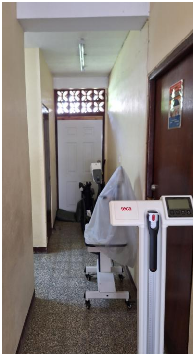
Figure 8-7: Showing Emergency Exit blocked by Medical equipment
