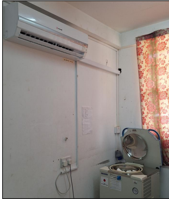
Figure 8-1: Showing AC Unit and Autoclave
