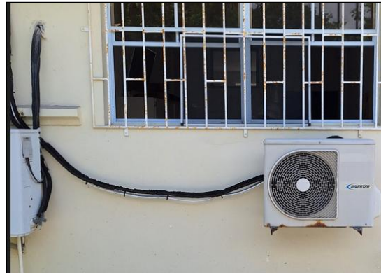
Figure 8-6: Showing Insulation on Copper tubing needs replacing
