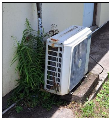
Figure 8-5: Showing Grass on the Condenser
