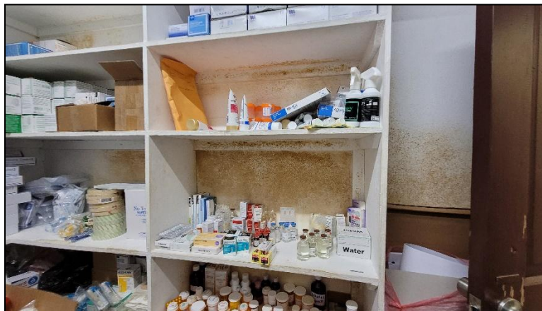
Figure 8-2: Showing Mould Growth in Storage Room
